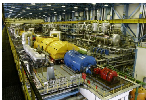
4 Turbine Hall of Paks
