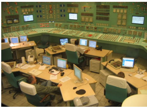
3 Control room in Paks
